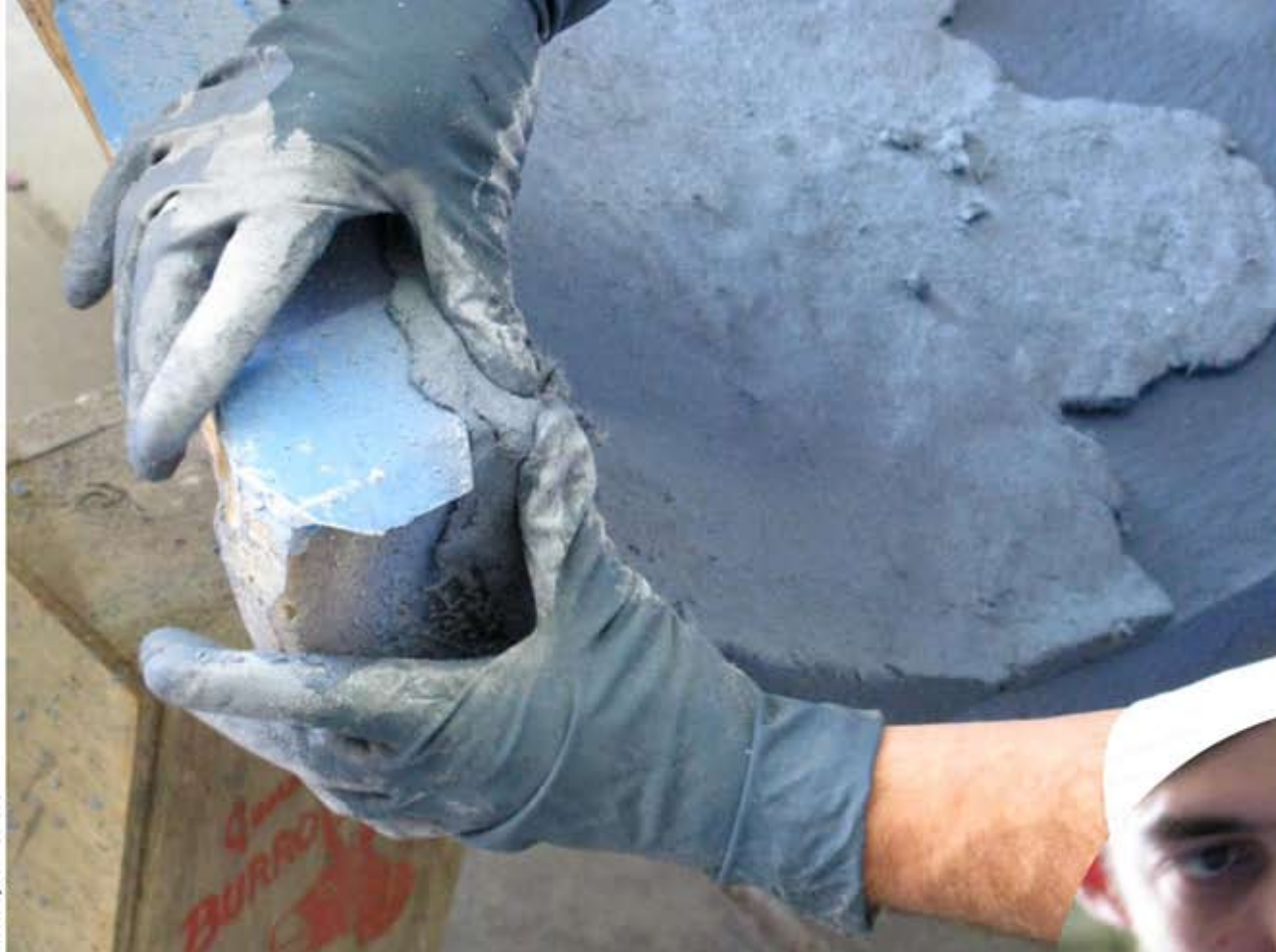
Left and below: Workshop participants hand-apply D-FRC at the Cheng Concrete warehouse in Berkeley, Calif.
