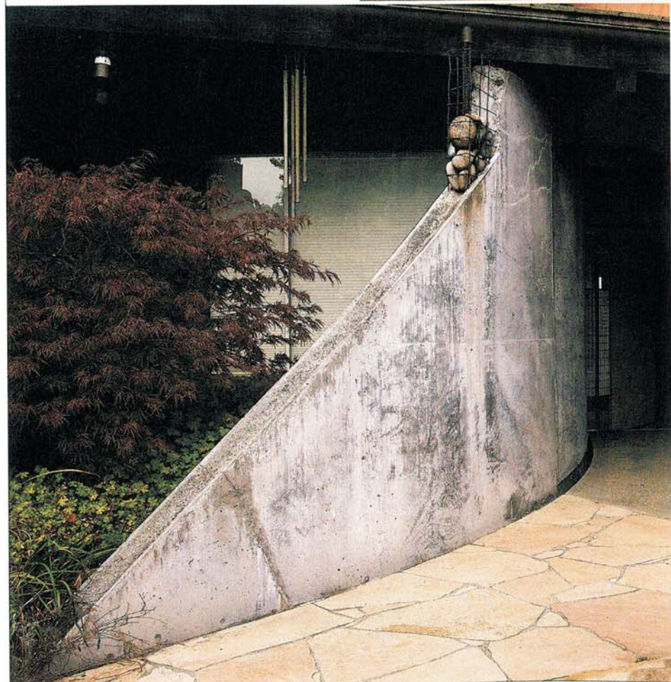
CHENG ON THIS MORAGA HOME'S WOOD STORAGE (ABOVE) AND STORM DRAIN (LEFT). RIGHT: MORAGA ABSTRACT.
